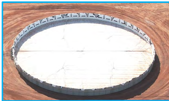
Typical Water Storage Tank
