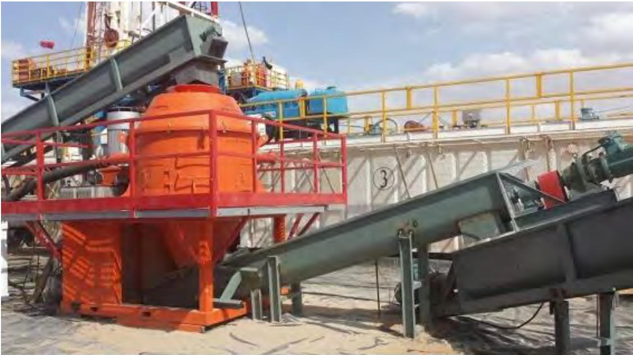
Figure 22: Example of a cuttings dryer used to recover synthetic based drilling fluids
