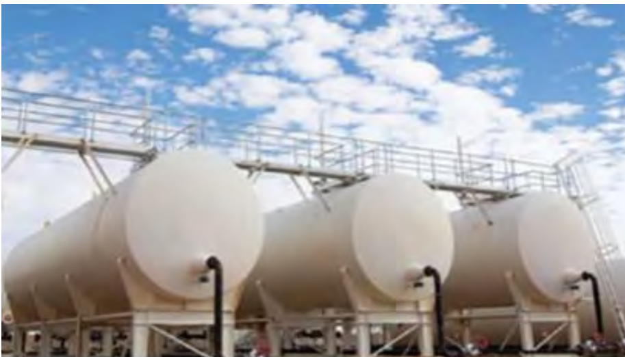
Figure 30: Example of condensate storage tanks (image provided for indicative purposes only)
