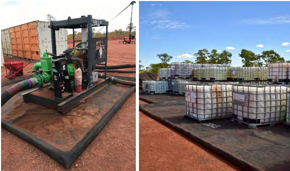
Figure 41: Examples of spill mats used to contain potential wastewater transfer spills
