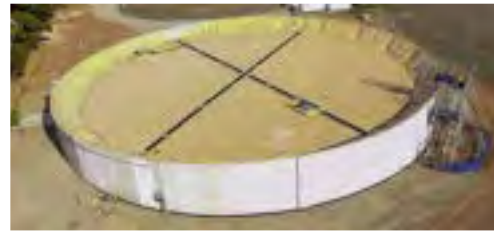
Image: Water/wastewater tank on wellpad with fitted cover
