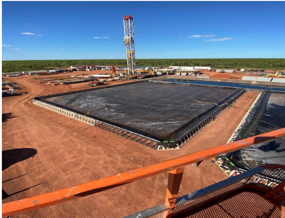
Figure 24: Covered water storage tank located on the existing Kyalla 117 N2 site
