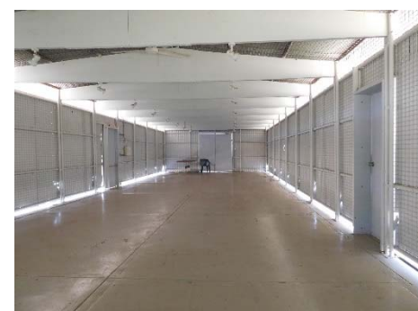
Fig.47 - Interior of the gallery space looking east. Walls are open top and bottom for ventilation. Ceiling fans are installed between truss members.
