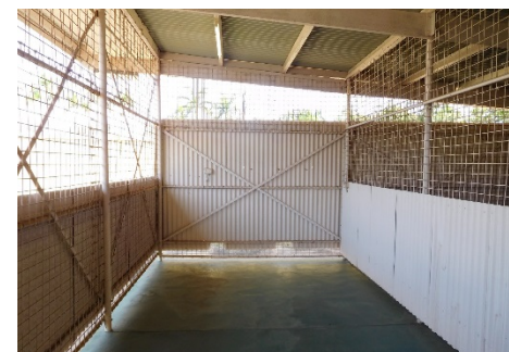
Fig.40 - Interior looking west. External walls to the north and south are weld-mesh above sill height. End walls are single skin with open gables.
