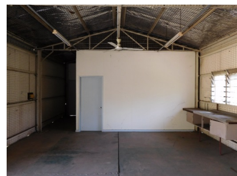
Fig.20 - Interior looking north. The CMP recommends removal of the later internal partitioning, removal of later louvre windows and reconstruction of the ventilation openings at the base and top of the external walls.
