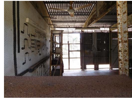
Fig.48 - Interior of the store area in the eastern side of the building. This area has weld mesh openings in the external walls and is well ventilated. Air conditioning outdoor units could be located within this space effectively concealing them from view.
