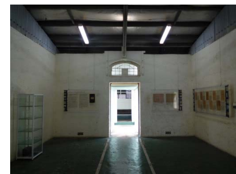
Fig.68 – Central area looking towards the passage to the Kitchen and Mess. A new door and frame is required and the highlight sealed.
