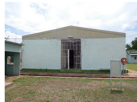
Fig.64 - East façade showing large barred door and screen to the central corridor.
