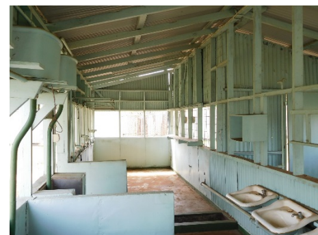
Fig.31 – Open interior of the Ablutions block. Note the open external walls and cladding to sill height only.
