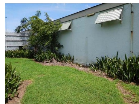
Fig.65 – North façade, western end, showing potential location for the outdoor unit in the yard between Cell block A and the Women's section.
