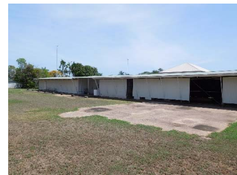
Fig.46 - Southern façade of the Stores building. The large opening is a door into the workshop
