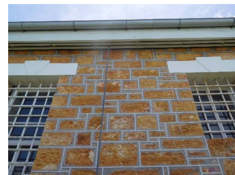
Fig.53 – External wall showing possible location for air conditioning refrigerant pipework running up to the roof space
