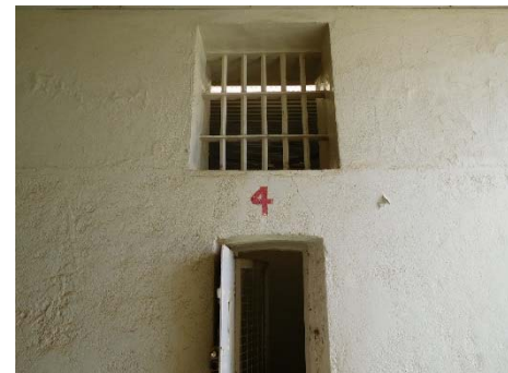
Fig.67 – Cell doors and large permanent ventilation opening above the door in the corridor wall
