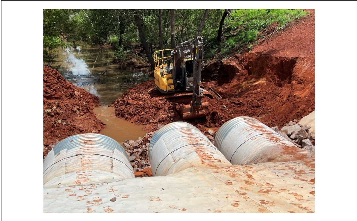
Plate 6 Development of erosion and sediment control works with culvert crossing in foreground
