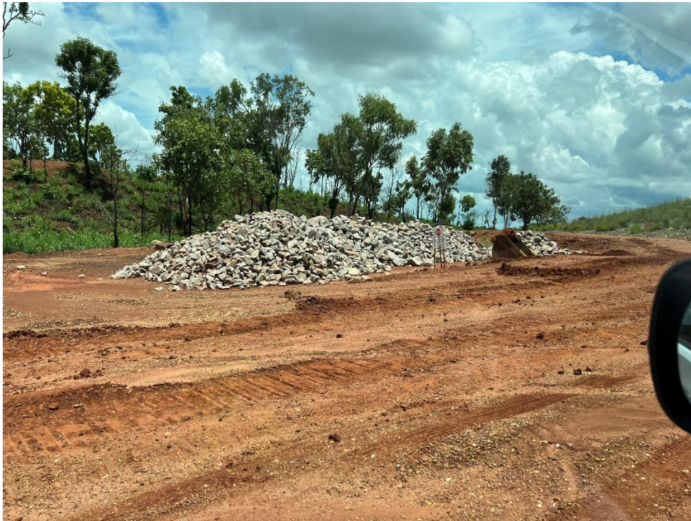
Plate 4 Rock stockpile for use in erosion and sediment control (culvert/diversion creek crossing works)
