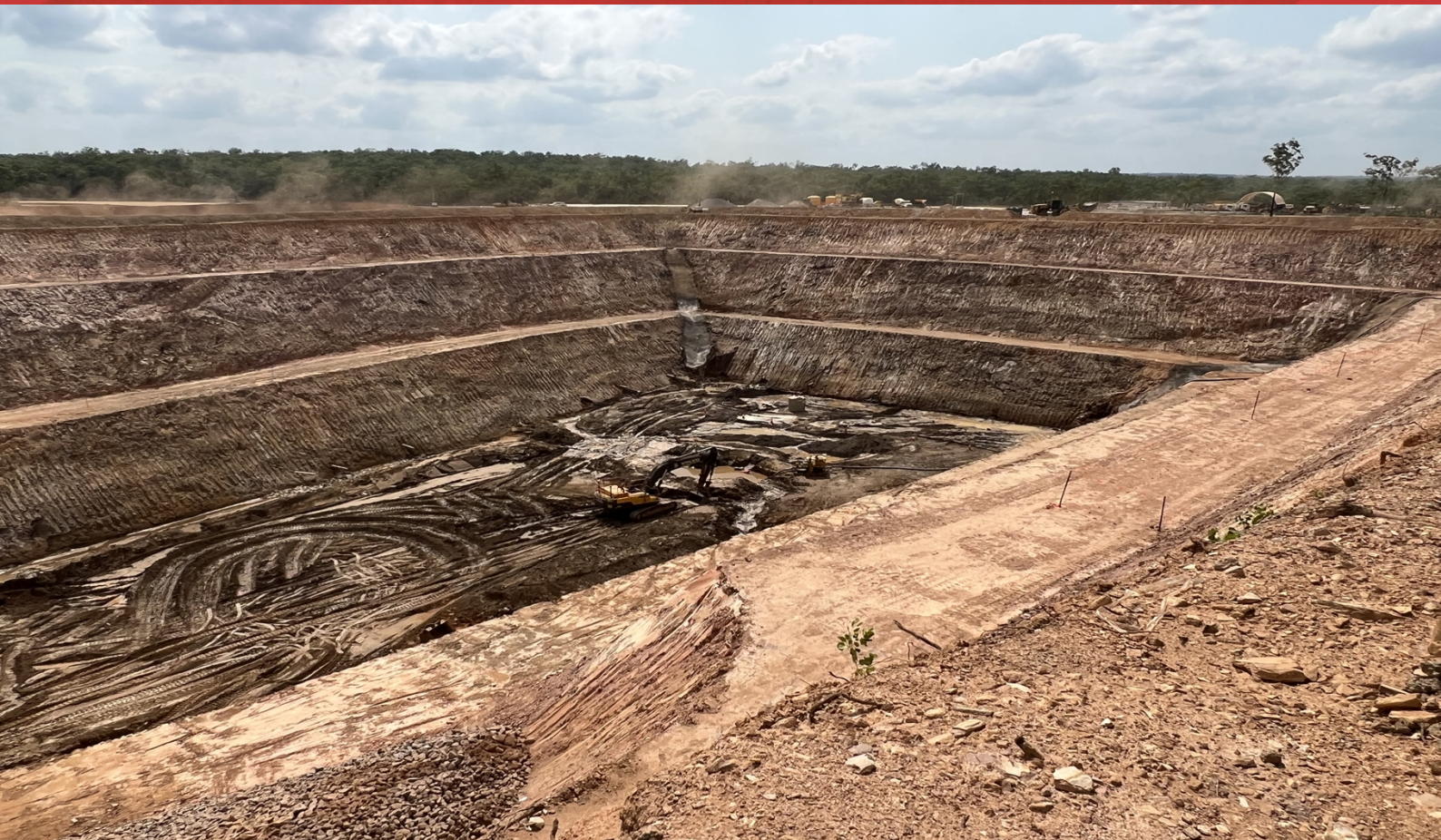
Image: BP33 Underground Mine Project during construction of box cut portal, October 2023
