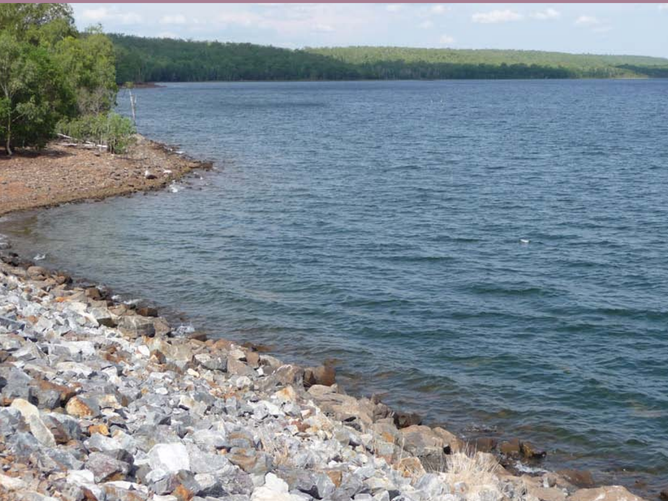
Darwin River Dam was constructed in 1972 and is designed to supply 200,000 people. Photo: John Drewry
