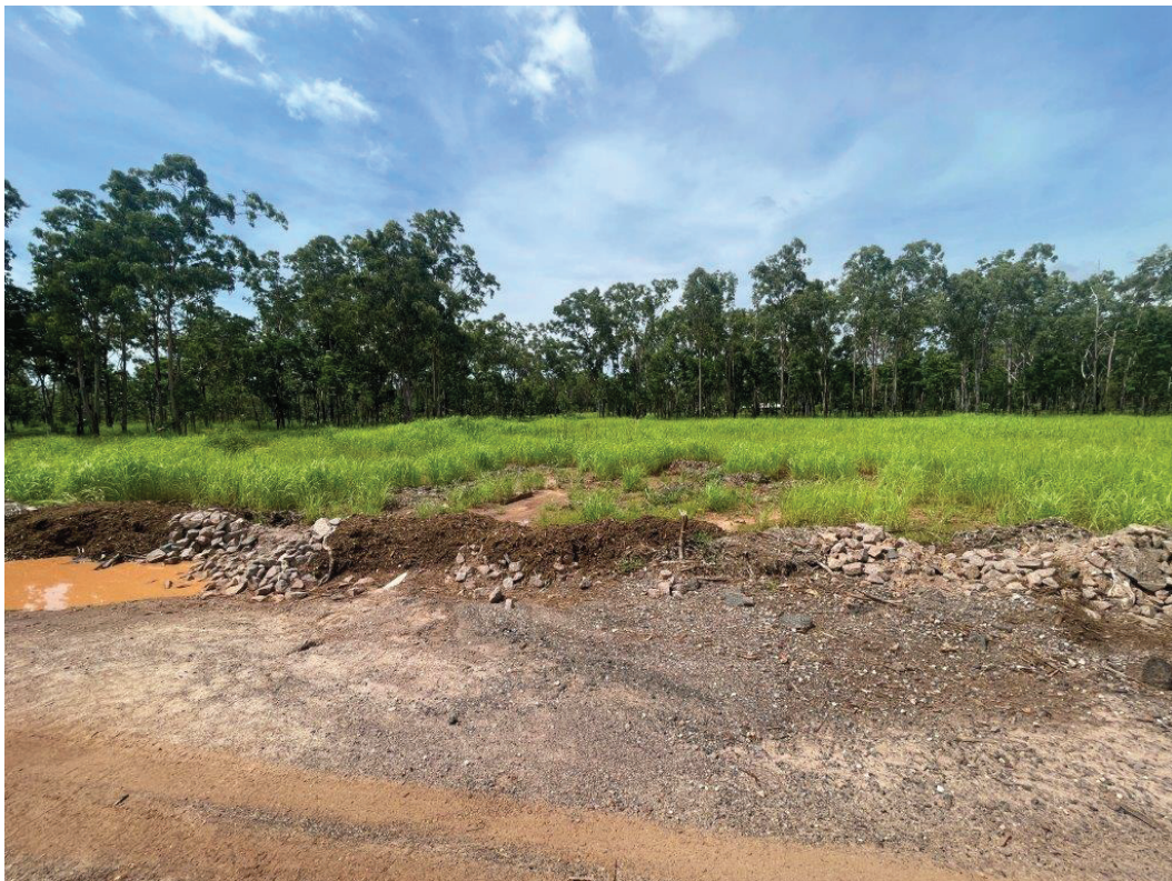
Dump Rock at Previous Breach in Mulch Berm. To be replaced with RFD.
