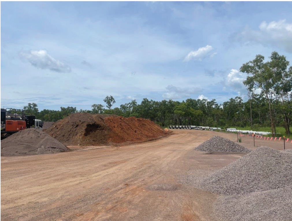
Compound with FCR Pavement. General Fill Stockpile without Sediment Controls.
