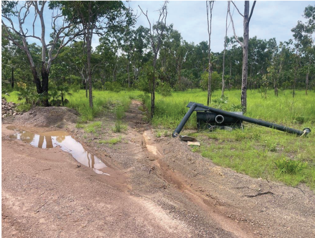
Typical Drainage Outlets on Western Perimeter of Compound Area.
