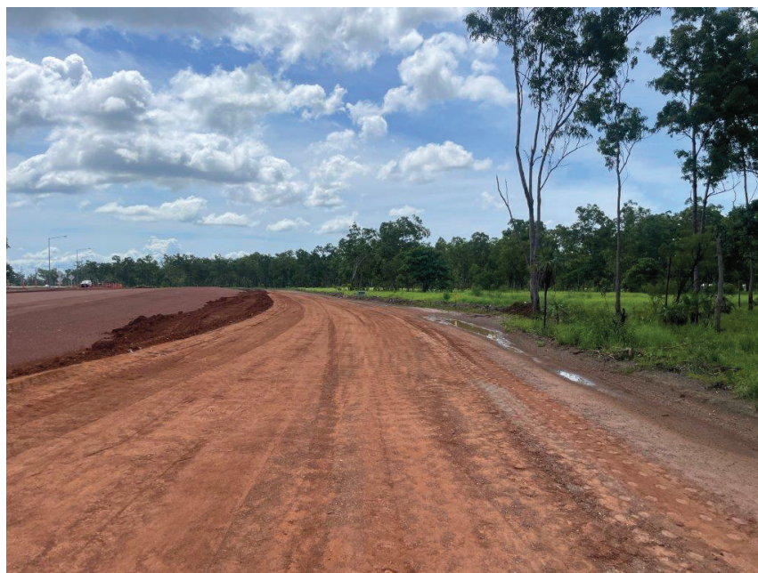
End of Mulch Berm approx. CH 550. Mulch Berm needs to be extended for full extent of works.
