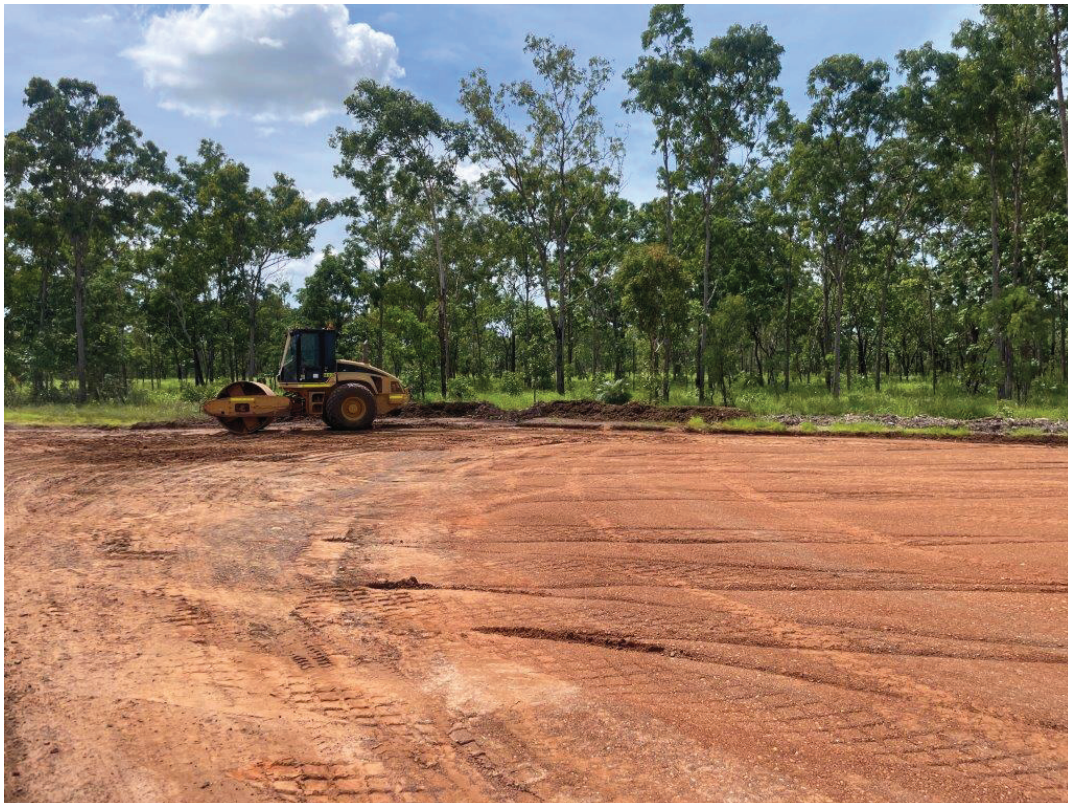
Start of Mulch Berm approx. CH 200. Flows are concentrating and dump rock has been installed where previous breach has occurred. Install Rock Filter Dam.
