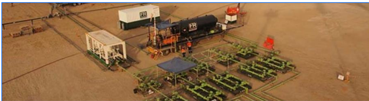
Figure 15: Separator package installed on a multiple well pad in Cooper Basin
