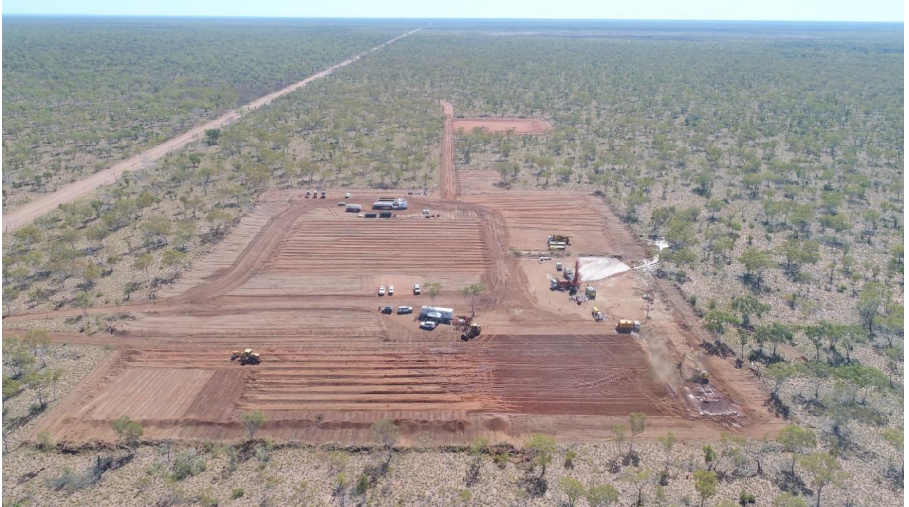
Figure 5 Overview of an exploration site within the Beetaloo undergoing lease and camp pad construction, with water bore drilling underway
