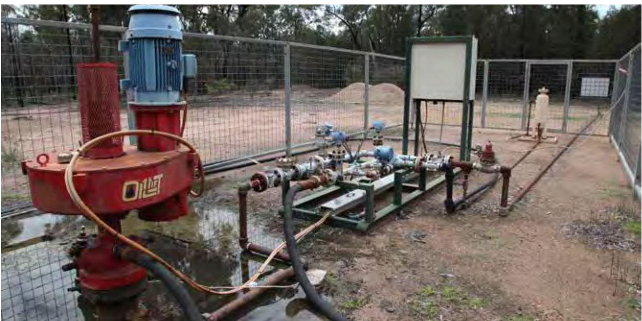
Decommissioned coal seam gas well, Pilliga Forest
