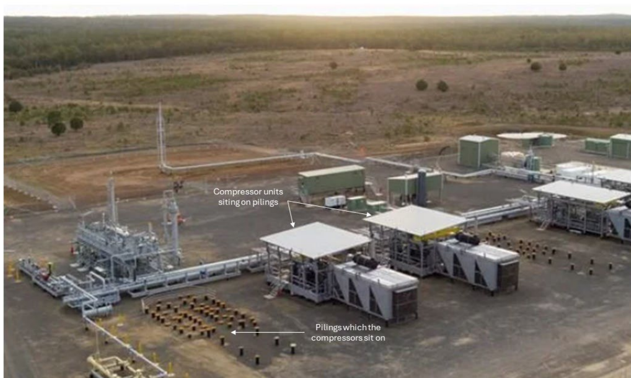
Figure 7: Example of compressor units with driven pilings
