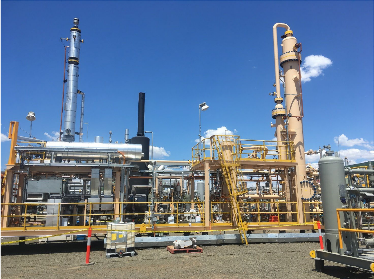
Figure 14: Example of a TEG unit (courtesy of GLP Group)
