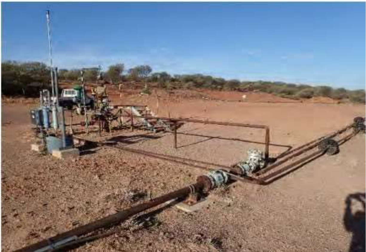
Figure 22: Typical well site layout and above-ground flowline
