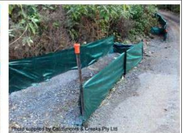
Photo 2 – U-shaped sediment trap within a mild gradient table drain
