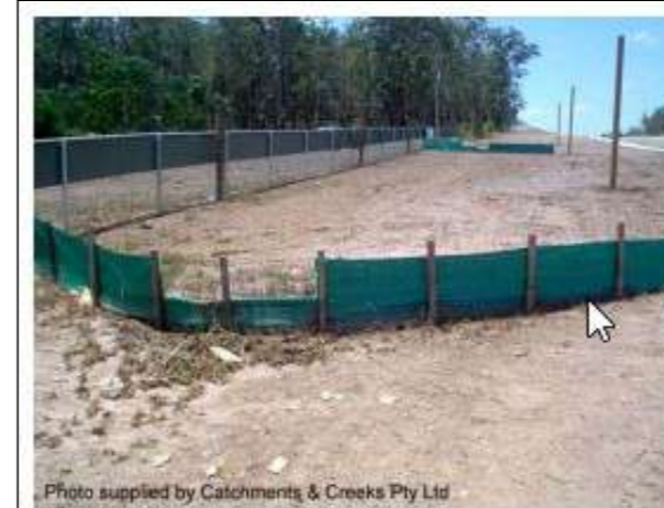
Photo 1 – U-shaped sediment trap within a wide drainage swale
