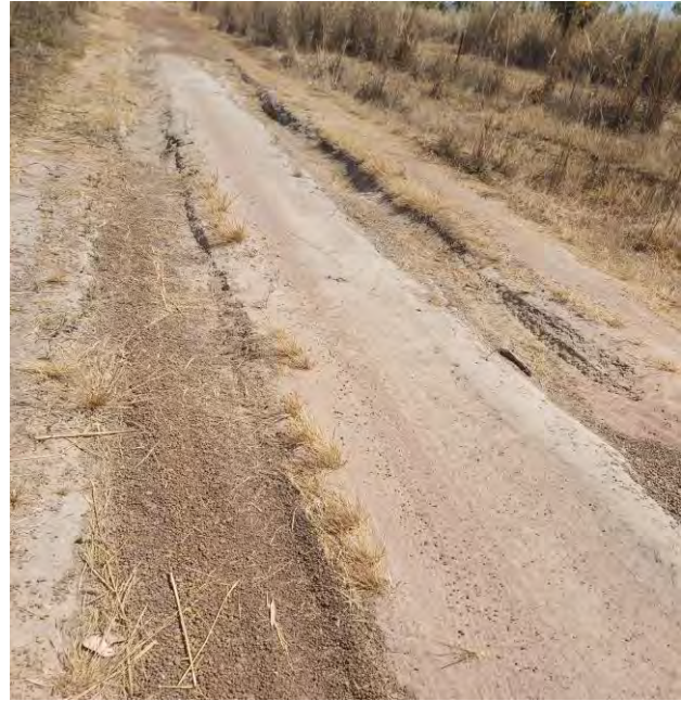
Photo 23 Acacia Gap Rd Northern side section 211 Note severe erosion, due to lack of maintenance
