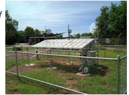
Artificial photosynthesis panels installed in Darwin, Australia
