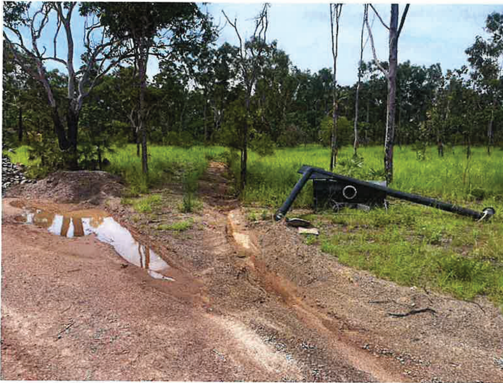
Typical Drainage Outlets on Western Perimeter of Compound Area.
