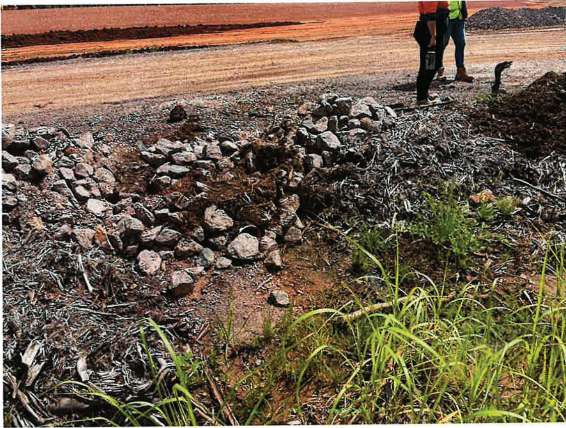
Uncontrolled PVC pipe outlet – 2 No. to be removed.
