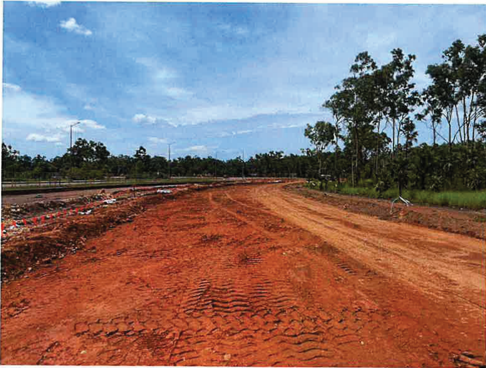
Dirty Water Catchment flows to Stormwater Pit DS3/5 or adds to Glyde Point catchment. Need to install diversion bank to convey water into Pit DS3/5 via Rock Filter Dam.
