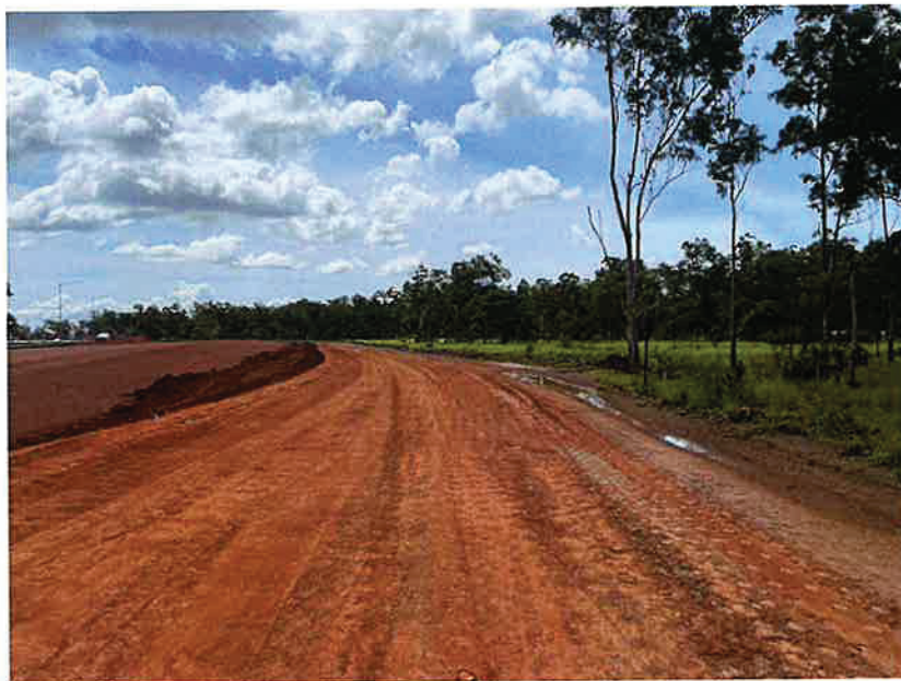
End of Mulch Berm approx. CH 550. Mulch Berm needs to be extended for full extent of works.
