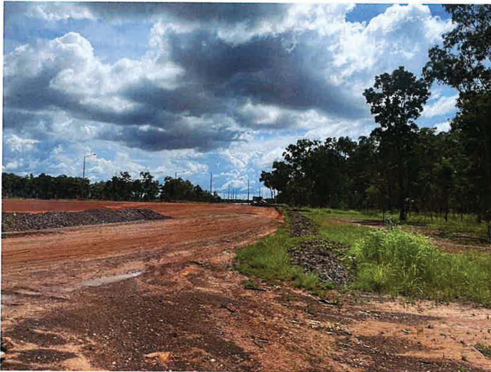
Gap in Mulch Berm for access track. To be closed off with a trafficable berm.
