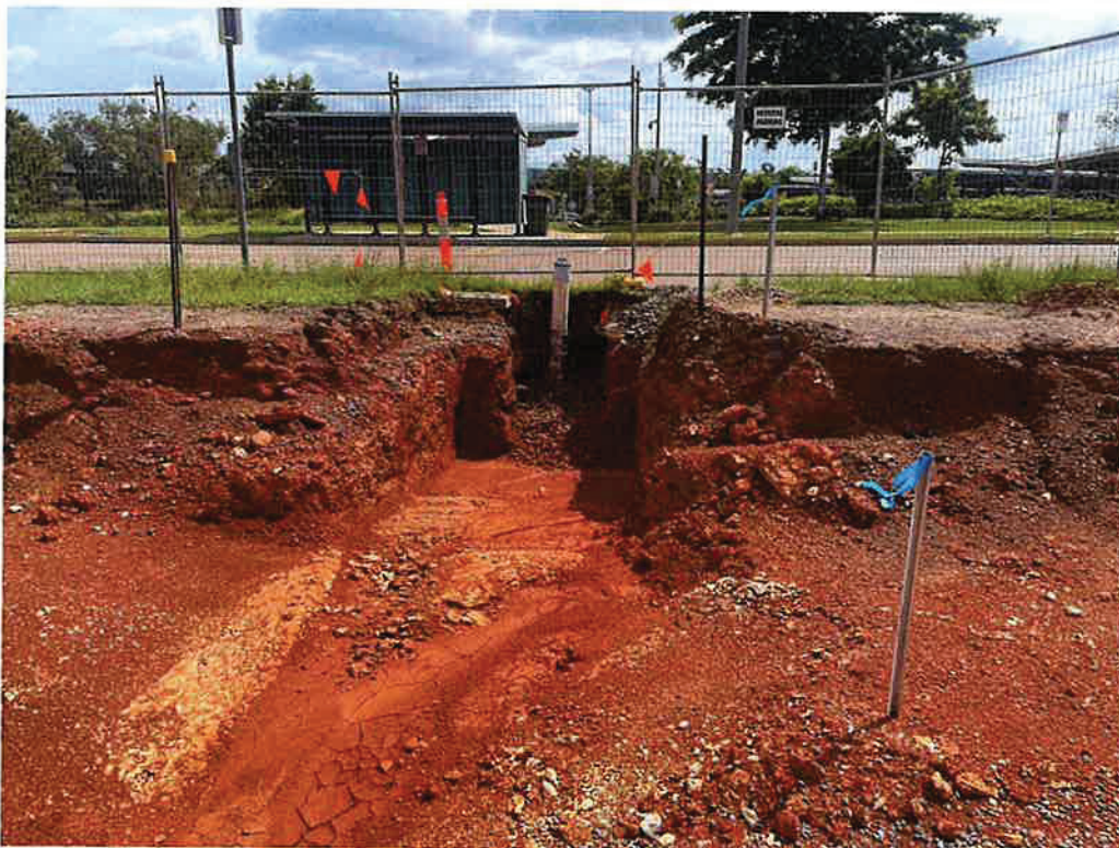
Filter rock and PVC riser to discharge stormwater into existing SEPs. Recommend addition of 500mm high RFD at start of trench (Typical).
