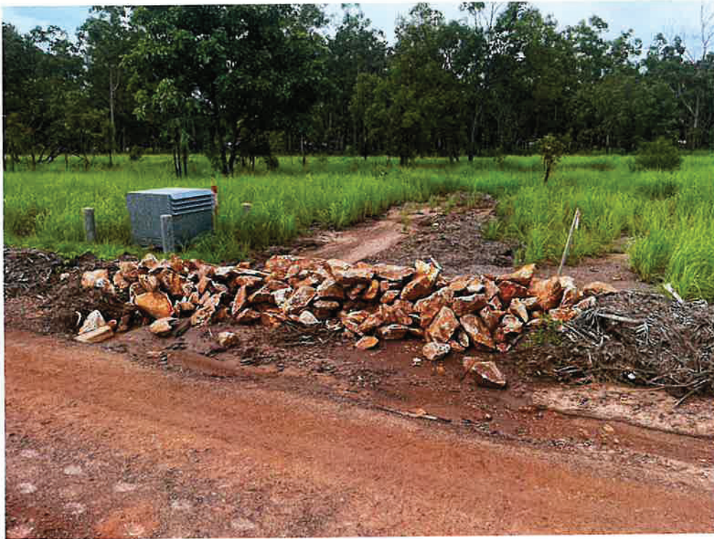
Dump Rock at Previous Breach in Mulch Berm. To be replaced with RFD.
