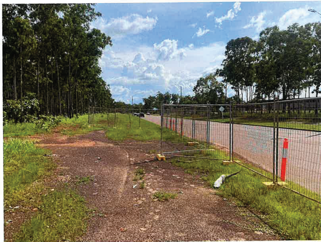
Sediment wash off onto PRH Access Road 2 from existing power track (appears historical)
