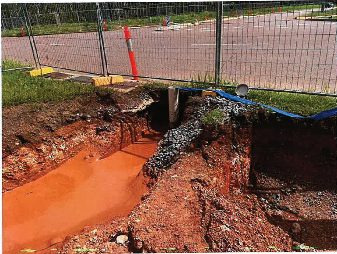
Dewatering Hose Connected to PVC riser without filtration measures.
