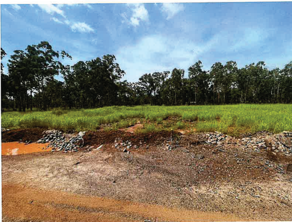
Dump Rock at Previous Breach in Mulch Berm. To be replaced with RFD.
