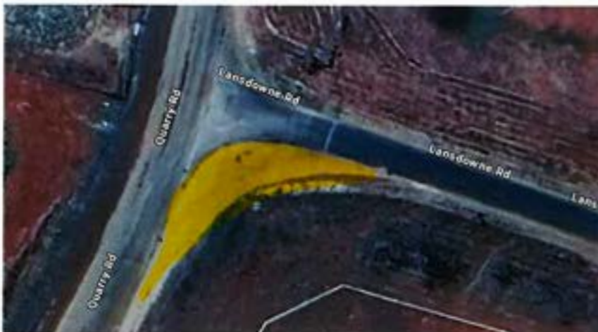
Image 1. Strain to highlighted area resulting from heavy vehicle usage of the Lansdowne and Quarry Rd intersection.
