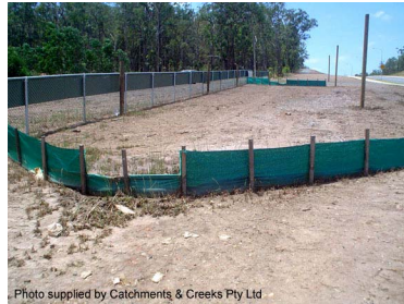
Photo 1 – U-shaped sediment trap within a wide drainage swale
